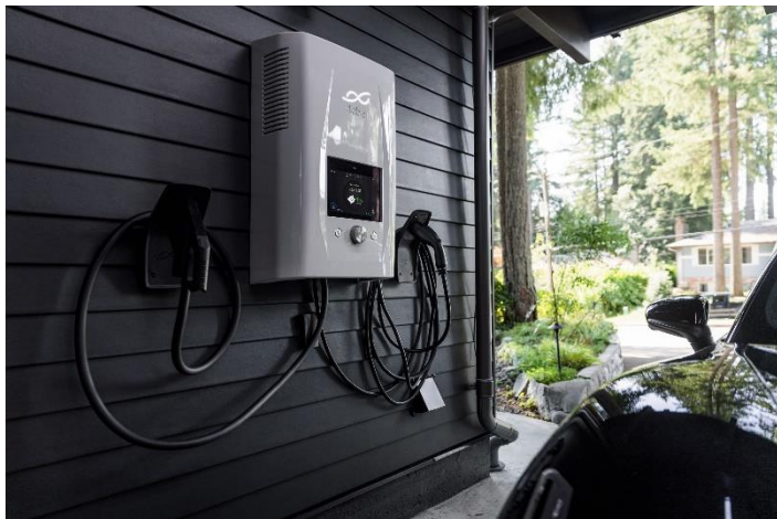
Indoor Charging Station
